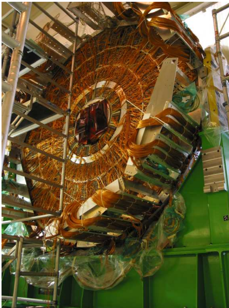
Figure 22. Photo showing the back face of the wheel with the special tools to bring the cable trays at their virtual position and the cables partially routed inside them.
